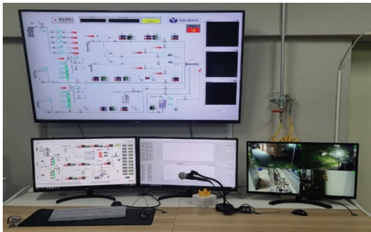
Fig. 6 Photograph of the control room.
