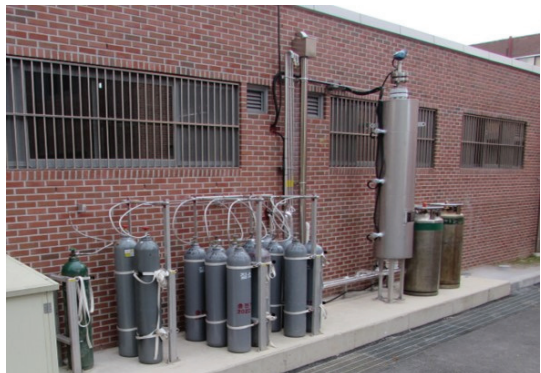
Fig. 3 LOx run tank and gas cylinder reservoir.
