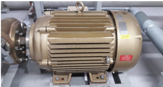
Fig. 4 Photo of liquid oxygen supply pump (K108-P40).
