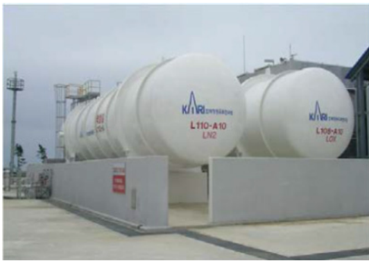
Fig. 3 Photo of liquid nitrogen (L110-A10, left) and liquid oxygen storage tank (L108-A10, right).
