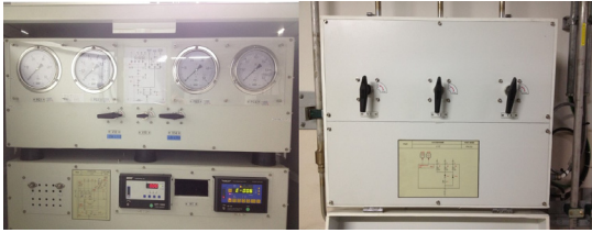
Fig. 3 Pumping rack and pumping valve unit.
